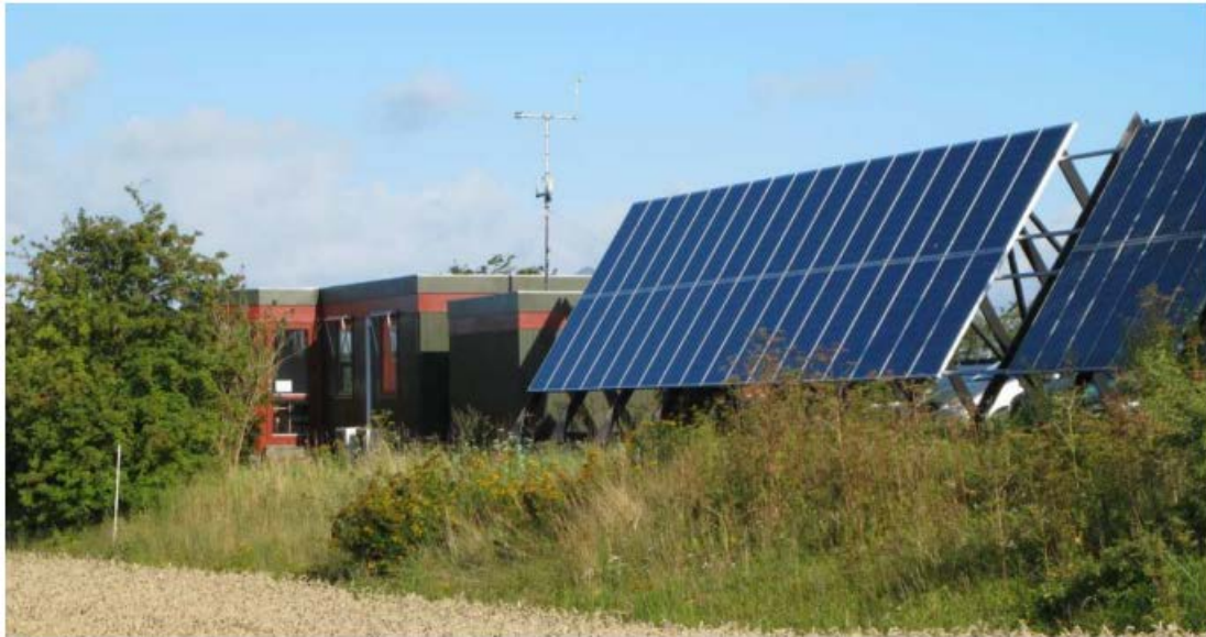
Figure 36: One PV plant located near building 715
